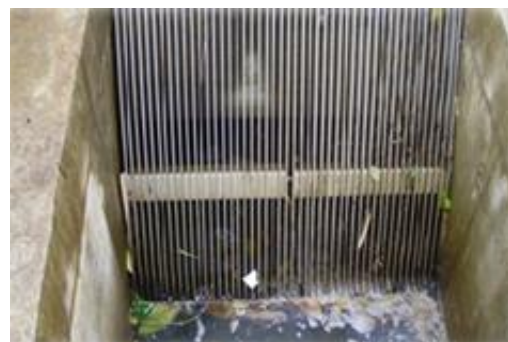
Figure 3 Screens of Intake
