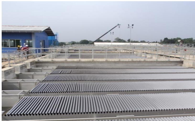
Figure 4 Flocculation Tank and Clarifier
