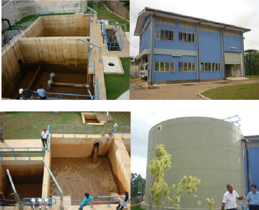
Figure 7 Sludge Treatment Unit
