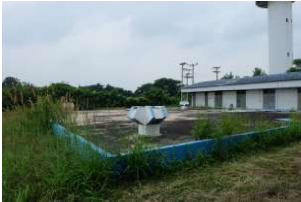
Figure 9 Clearwater tank at Paisadao WTP
