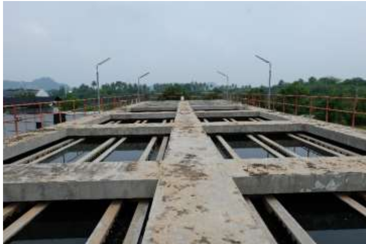
Figure 7 WTP sedimentation basins
