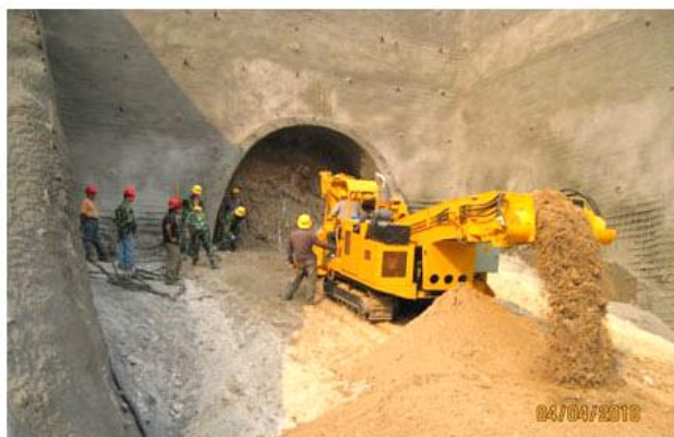
Figure 1: Excavation of tunnel to divert raw water from Melamchi (Melamchi Water Supply Development Board, 2013)
