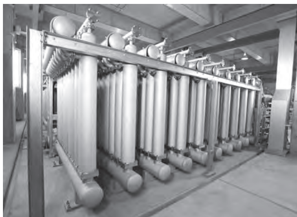
Ceramic membrane filtration system in the plant
