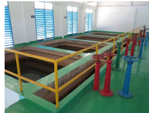
Manual operated valve (1 st WTP)
