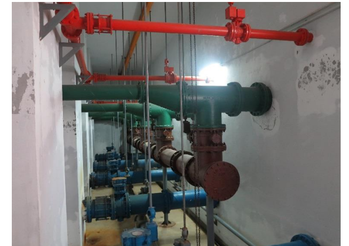
Identification of Pipe Line
