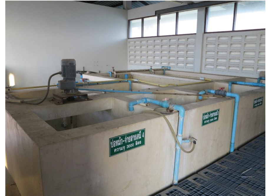
PAC Solution Tank
