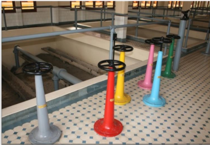
multiple colored pipeline valves system
