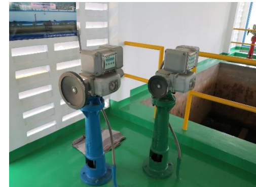
Motor-operated valve (2 nd WTP)
